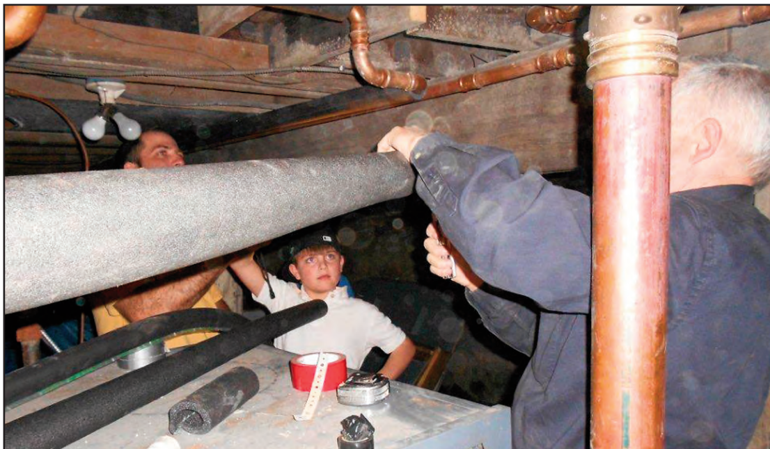
Colby Stewart holds insulation in place while his father, Mark, and Tim White take measurements.
